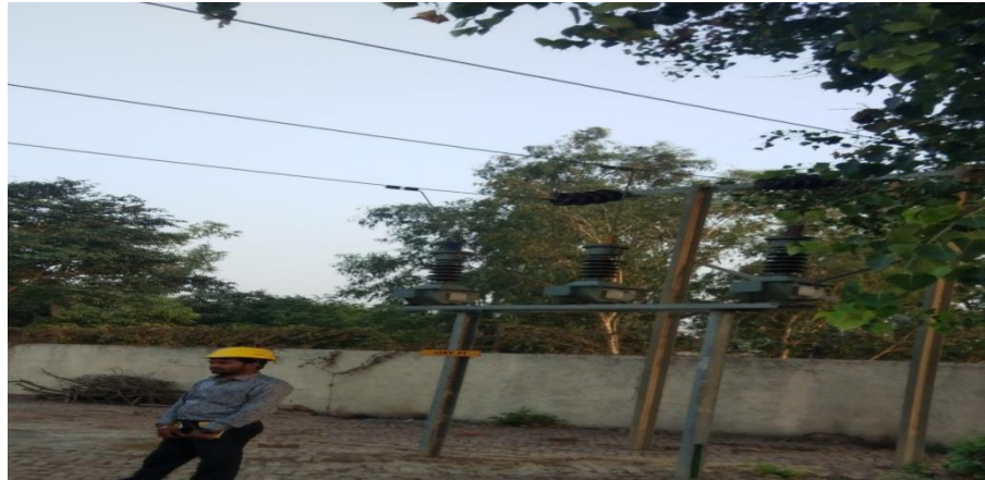
Fig 7: Bus bar at sub station.
