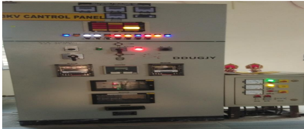
Control relay Transformer panel
